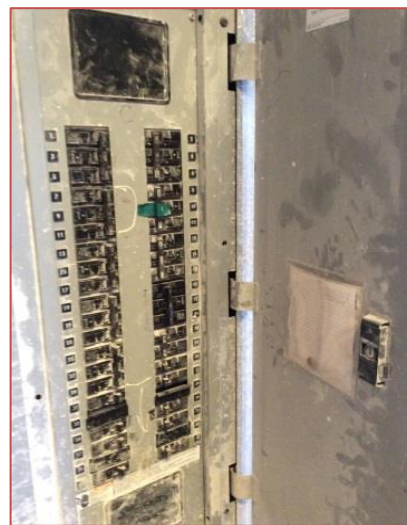
Purpose of Individual Breakers Not Marked or Listed
