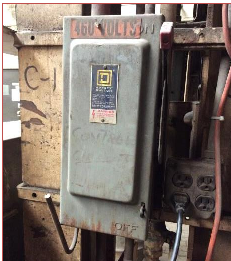
Markings on Disconnecting Means No Longer Legible
